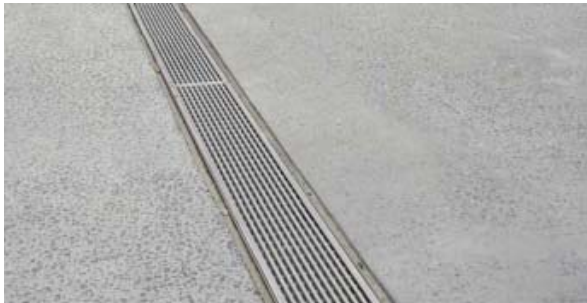
Stainless steel trench grate for concrete pavement
